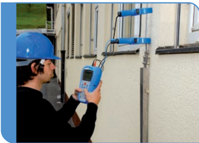
Two clamps method for testing ground resistance of object on TN system
